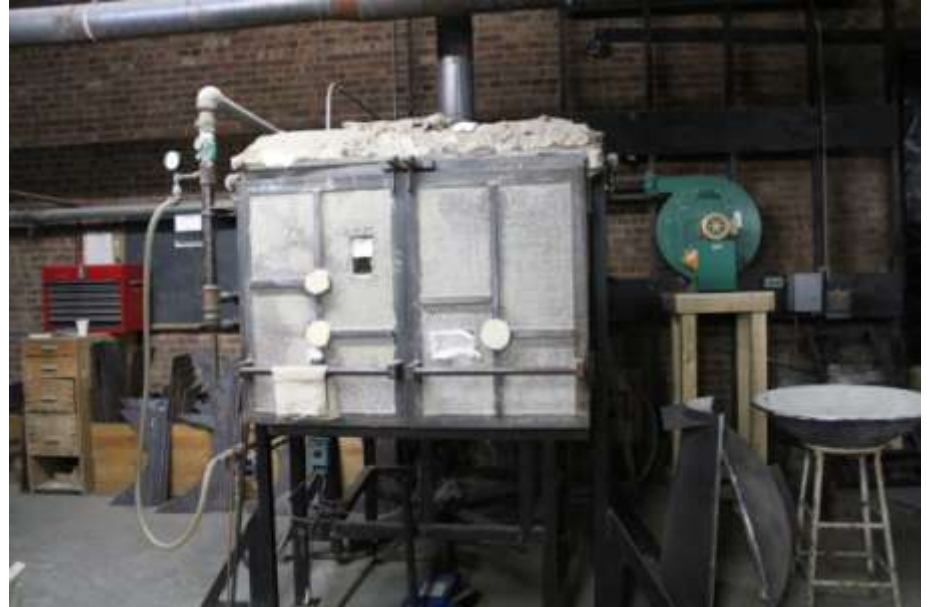
Five at-risk custom kilns; this one features newly elevated electrical engine to the left of the kiln.
