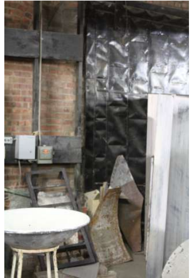
Connecting door between leased units allows water to enter Flickinger production area.
