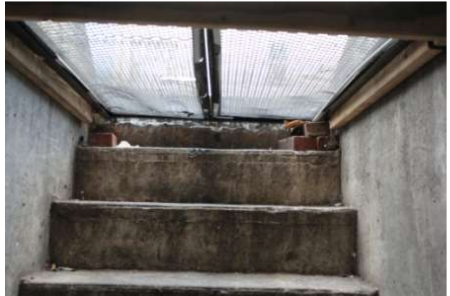
Temporary mitigation opportunity: fabricate temporary flood barrier to fit hatch frame. Install barrier and seal joints with spray foam.
