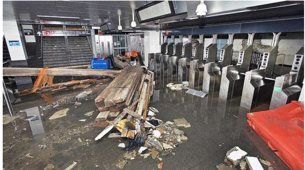
Post Sandy flooding of MTA subway station
