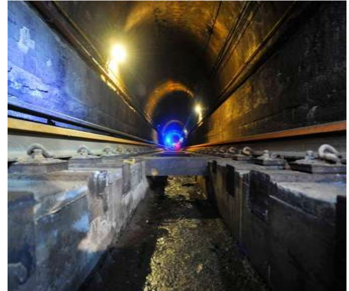
Super storm Sandy flood water receding from MTA R line tunnel
