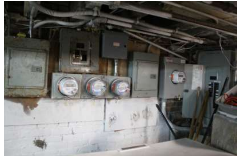
Electric service entrance in basement Meters for Fort Defiance Café and 2 nd and 3 rd floor tenants
