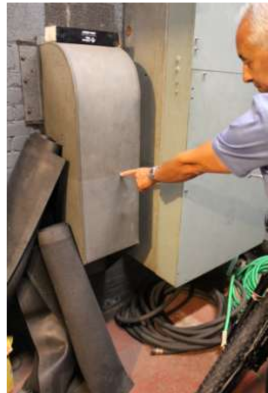
High water mark in mechanical/electrical switchgear room
